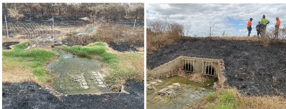
Photos 1 – 2: Unauthorised Discharge to Receiving Environment
